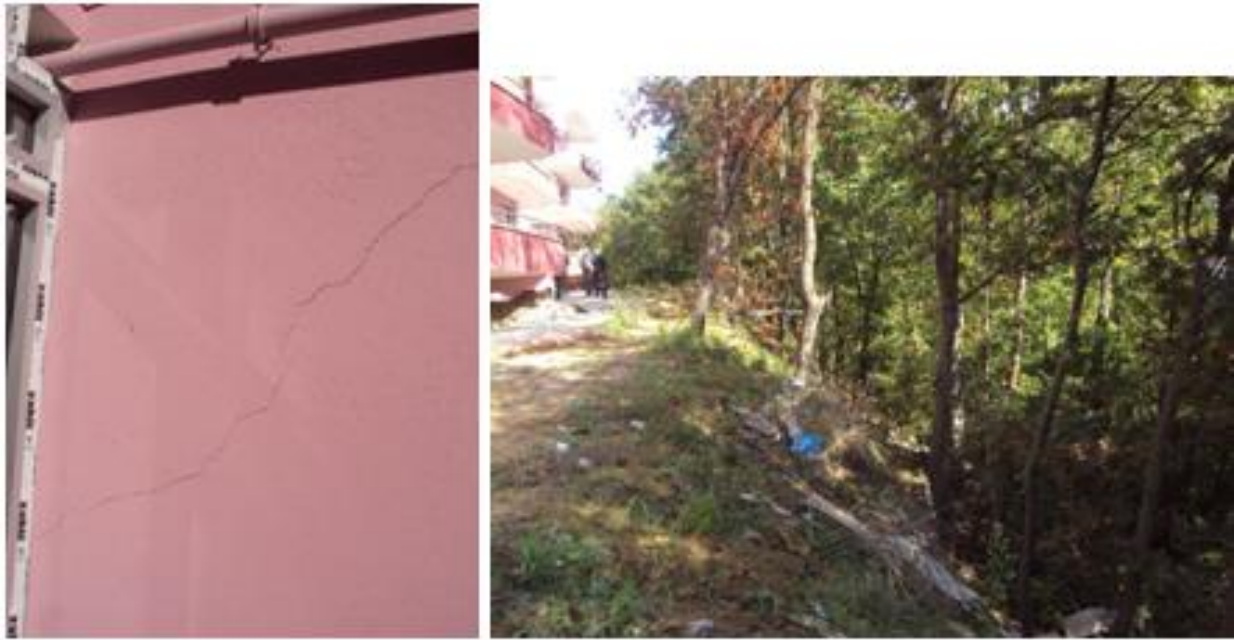
Figure 2. Settlement crack and filling on the slope
